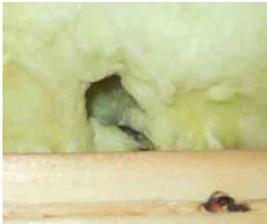
Figure H: Rodent hole through insulation
