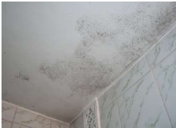
Figure F: Mould on ceiling
