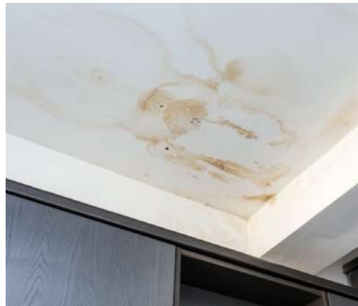
Figure B: Brown water stain
