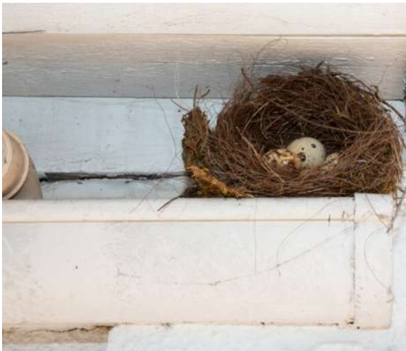
Figure J: Nest in gutter
