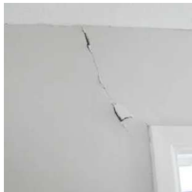
Figure D: Crack in wall due to water ingress
