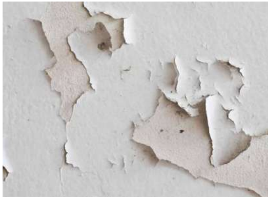
Figure E: Water damage causing paint to peel
