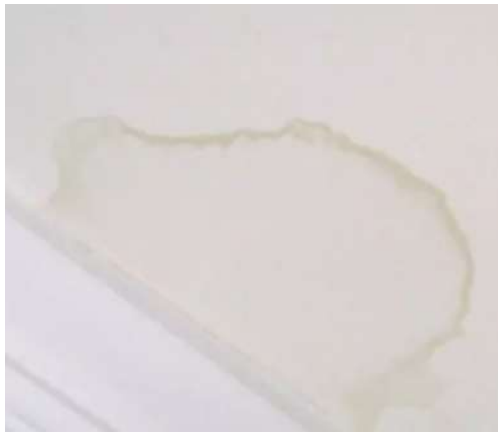
Figure A: White/yellow water stain
