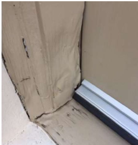
Figure F: Paint peeling due to termites
