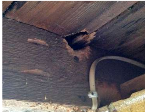
Figure D: rodent hole
